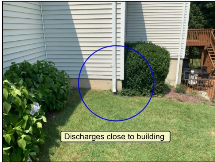
Discharge too close to building
