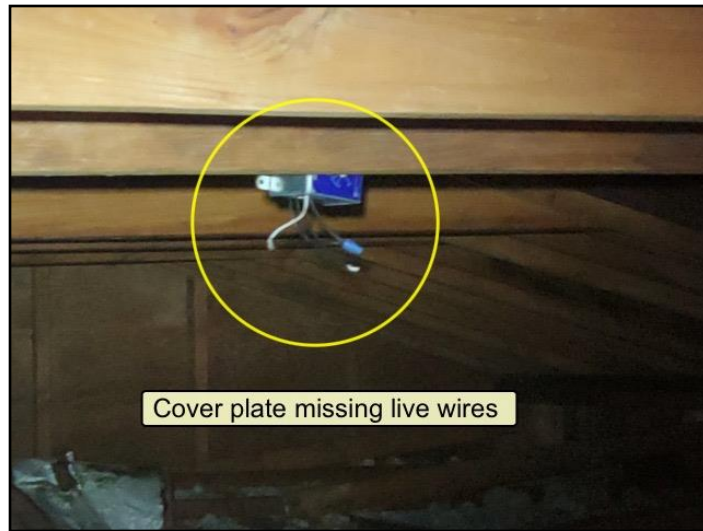
For junction box is missing
